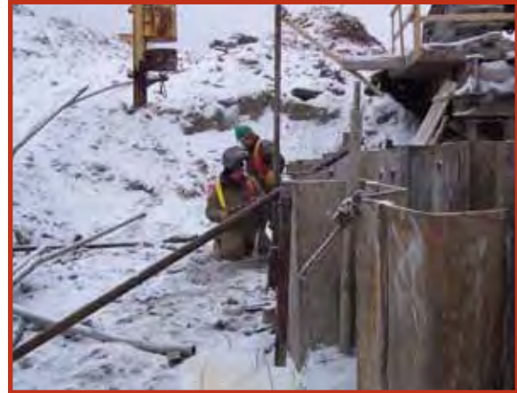
Agnico-Eagle, Goldex, Quebec Construction of a shaft collar through quick sand was overcome using a systematic engineered grout plan. The plan specified strategic placement of grout pipes as well as appropriate cement grout mixture for this unique application.
