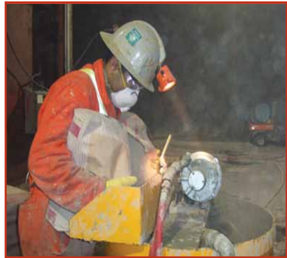
Sifto Salt, Goderich Mine, Ontario Chemical grout, applied as spray foam, was used to seal a five meter high by eight meter wide underground ventilation bulkhead. A layer of cement grout (in the form of spray foam) was applied over top for fire protection purposes.
