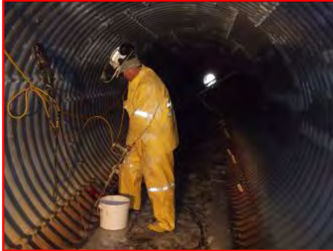
RIGID GROUT is used to fill voids in culverts beneath an airport runway. Repairs were required to prevent settlement.
