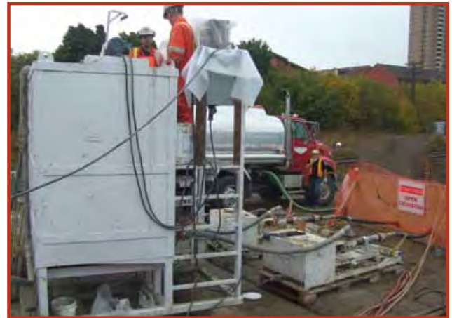
Utility Services, Cellular Grouting, Toronto, Ontario Light weight cellular grout is used to backfill casings after delicate conduits and high voltage cables are installed beneath railroad tracks, airport runways or roadways.
