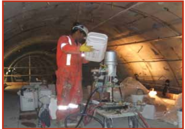
Tunnel Construction, Chemical Grouting, Edmonton, Alberta Chemical grout is used to stabilize soil, cut off active water flow and seal leaking joints in various forms of tunnel construction.
