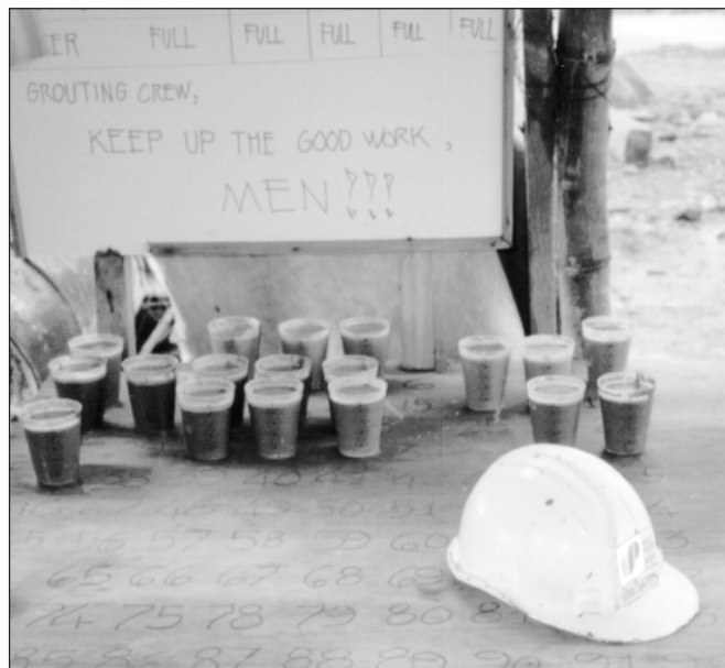
FIGURE 9 - QUALITY CONTROL STATION
