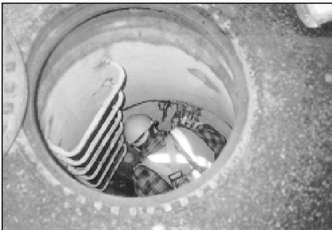
Precast manholes are permanently sealed with MULTI-GEL resin, using special manhole sealing equipment and injection techniques supplied by MULTIURETHANES
