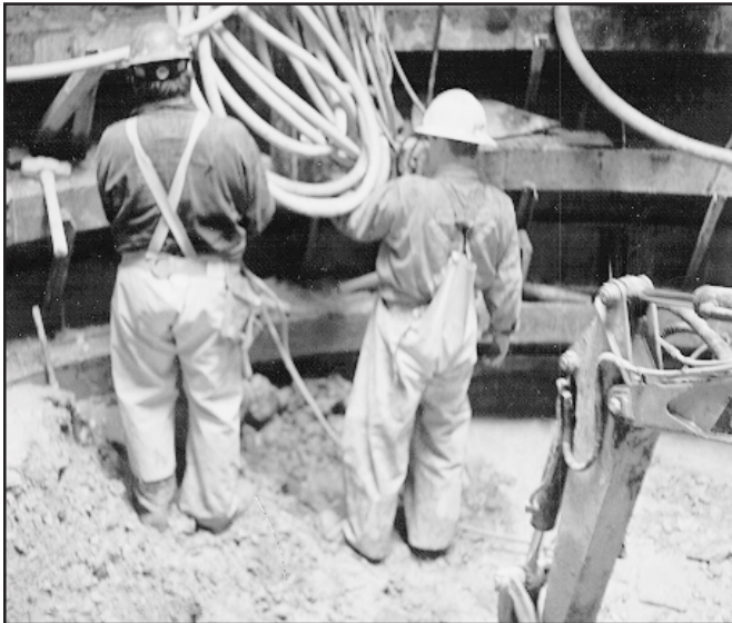
Miners preparing for polyurethane injection to stop inflows of quicksand into a 24 foot diameter shaft collar excavation
