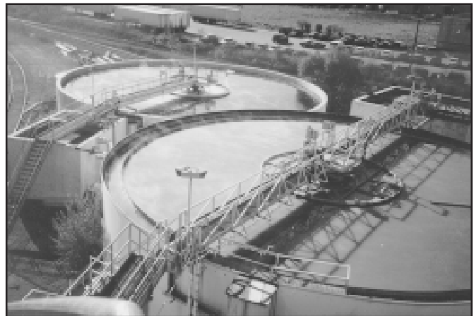
Cracks in concrete water treatment tanks are sealed from the outside while the tanks remain in operation using MULTIURETHANES injection products, equipment and accessories
