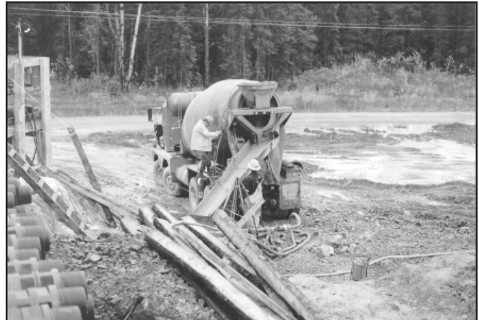
For large scale grouting operations, ready-mix plants can be used to supply bulk grout formulations at substantially lower costs than site-mixed grouts
