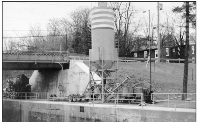
Large grouting jobs such as this lock rehabilitation project utilize bulk cement delivered into on-site storage silos with integral auger feed screws to deliver cement into the colloidal mixer on a demand basis.
