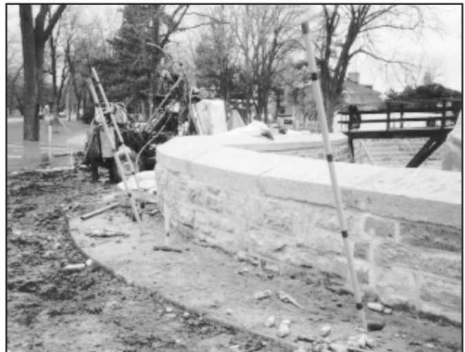
Sleeve pipes installed beneath masonry walls of an old fortification originally constructed in the early 1800's; scope of work utilized microfine cement grouts to reduce permeability within masonry structure.
